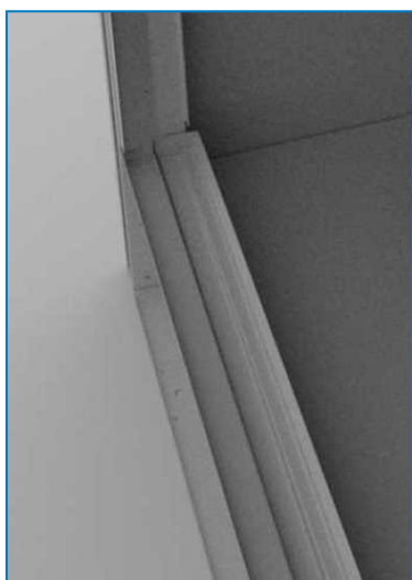
Water collection gutter
