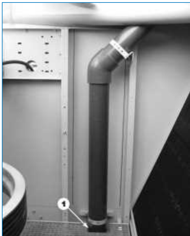
Pump piping plenum section inside
