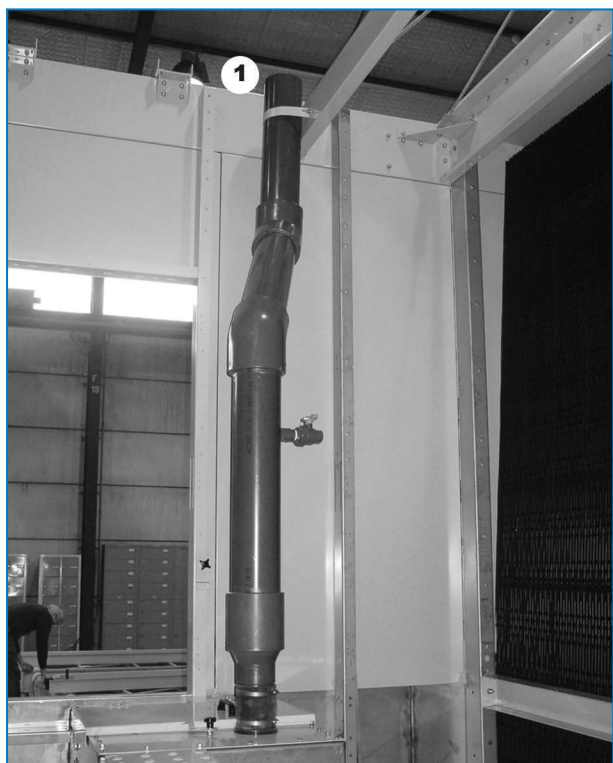
Pump piping lower section
